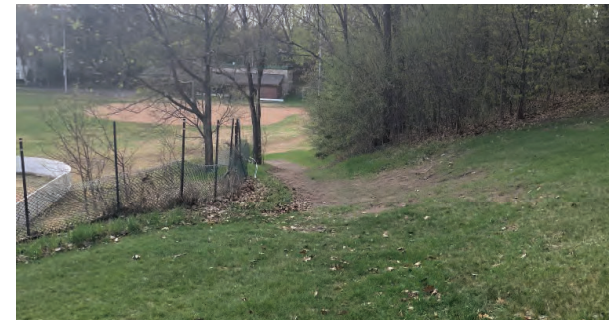
Existing hillside showing erosion on non-accessible route.
